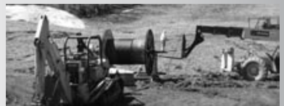
The wire rope is spooled up. It will be re-used on the new lift.
